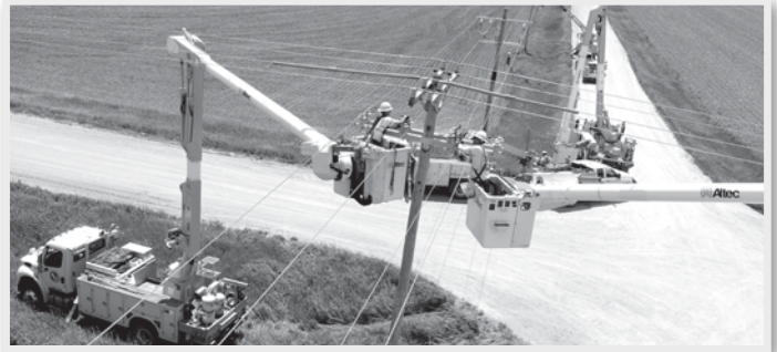
New three phase line construction our crews worked on this past summer
